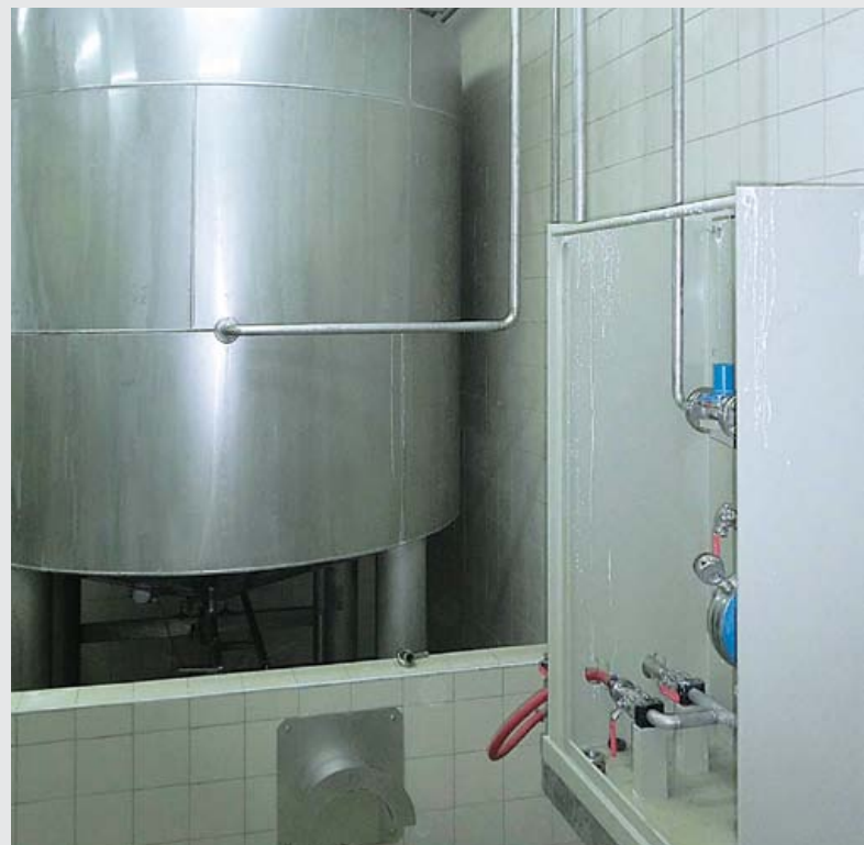
sera transfer unit and storage tank for the prepared solution
