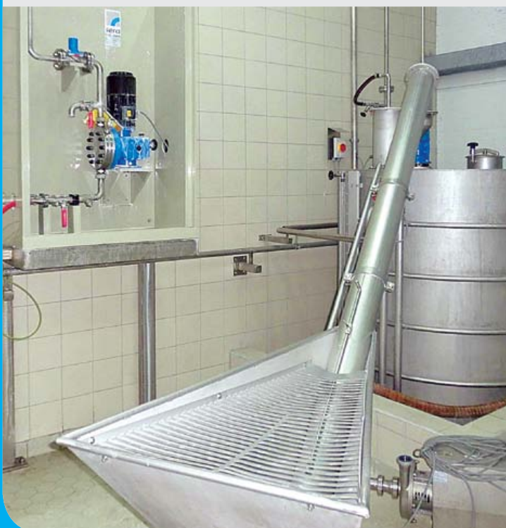
The sera transfer unit (left) transfers the prepared solution from the integrated preparation tank (right) into a separate storage tank
