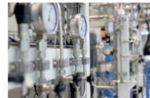
Precise measurement and control technology: instruments that guarantee maximum purity and process reliability in CO 2 compression.
