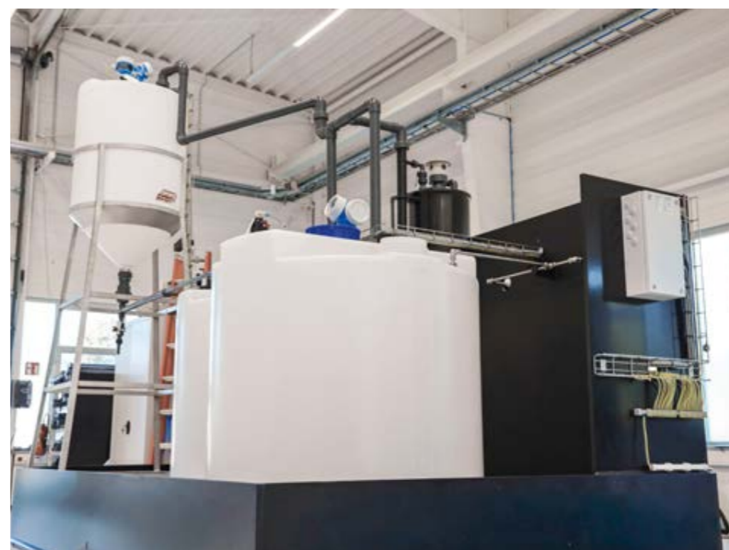
Dilution station for ammonia with storage tanks: dilution of 25% ammonia to 0.5 to 2% ammonia and storage in two storage tanks.
