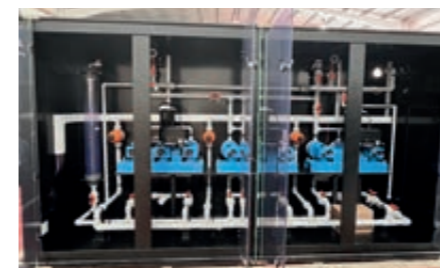
Dosing system for sodium hypochlorite: It consists of three triple pumps (two in operation, one in reserve). The sodium hypochlorite is injected into the seawater for disinfection before it enters the reverse osmosis process.
