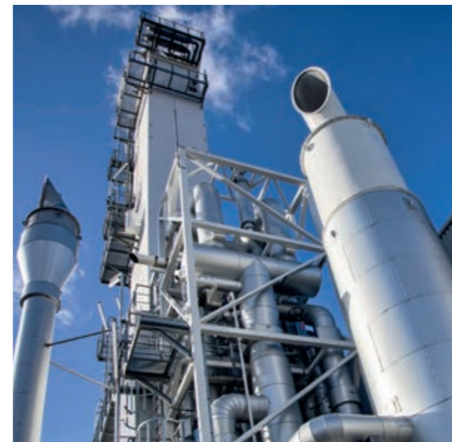
Modern air separation plant from SWF at the Bielefeld site.
