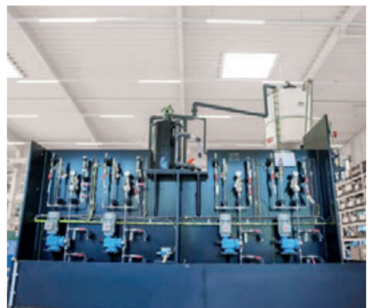
Rear of the dosing station for caustic soda.
