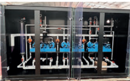
Dosing system for sodium hypochlorite: It consists of three triple pumps (two in operation, one in reserve). The sodium hypochlorite is injected into the seawater for disinfection before it enters the reverse osmosis process.
