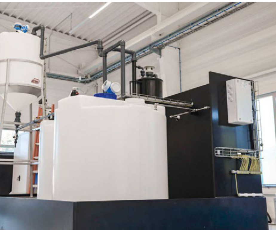
Dilution station for ammonia with storage tanks: dilution of 25% ammonia to 0.5 to 2% ammonia and storage in two storage tanks.
