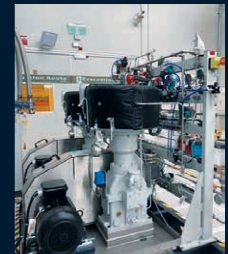
Clearly visible in the image: The (black) insulation of the electrically heated valve heads and the arrangement of the redundant compressor stages.
