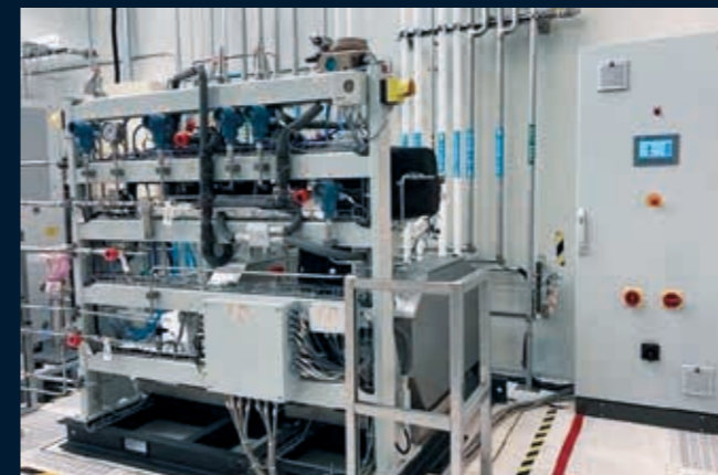
Instrument rack and control cabinet for controlling the two metal diaphragm compressors of type MV3 at our Taiwanese customer.
