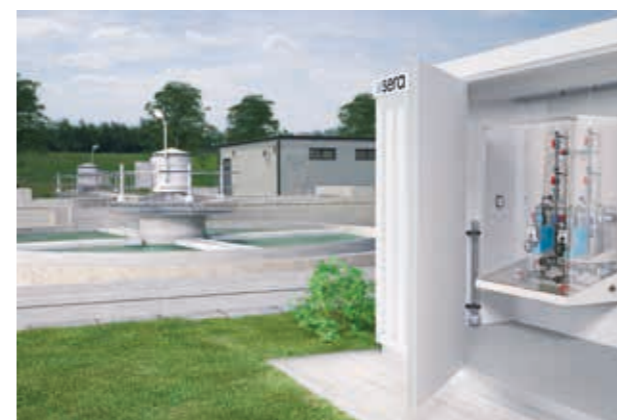
sera container solutions in use in municipal sewage treatment plants.
